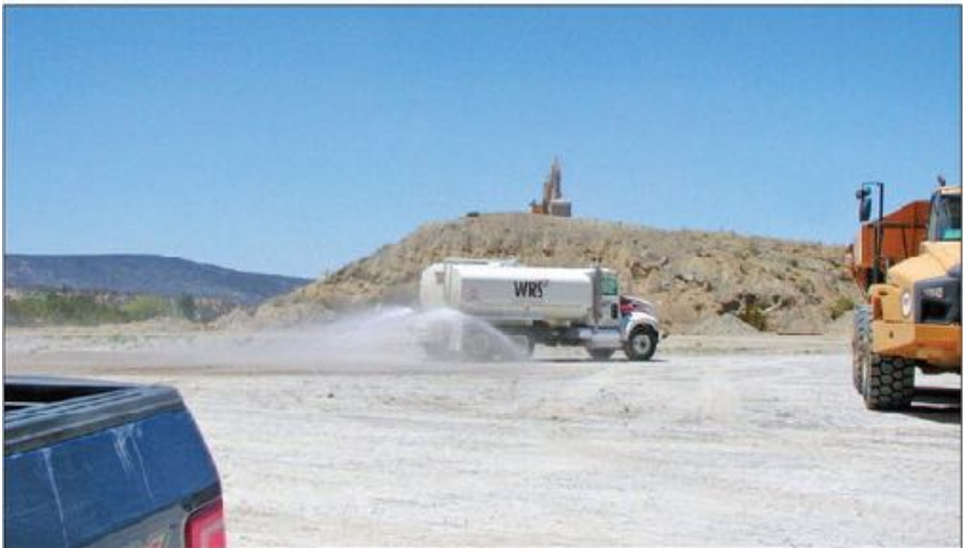
Water is sprayed on the roadway to eliminate fugitive dust while work is conducted at the Mount Taylor Mine.
